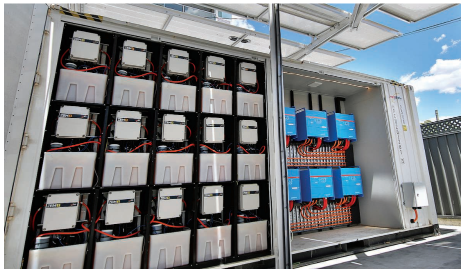
Commercial flow batteries, such as this zinc-bromine system from Redflow, are helping back up renewables.
